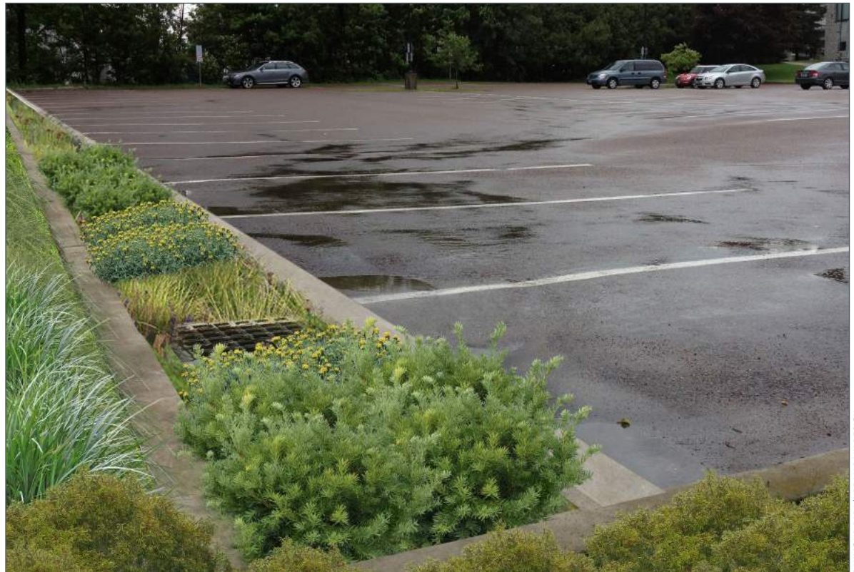
▲ RETROFIT OPPORTUNITY: The same parking lot scenario replacing the first couple of feet of asphalt with a green gutter system.
