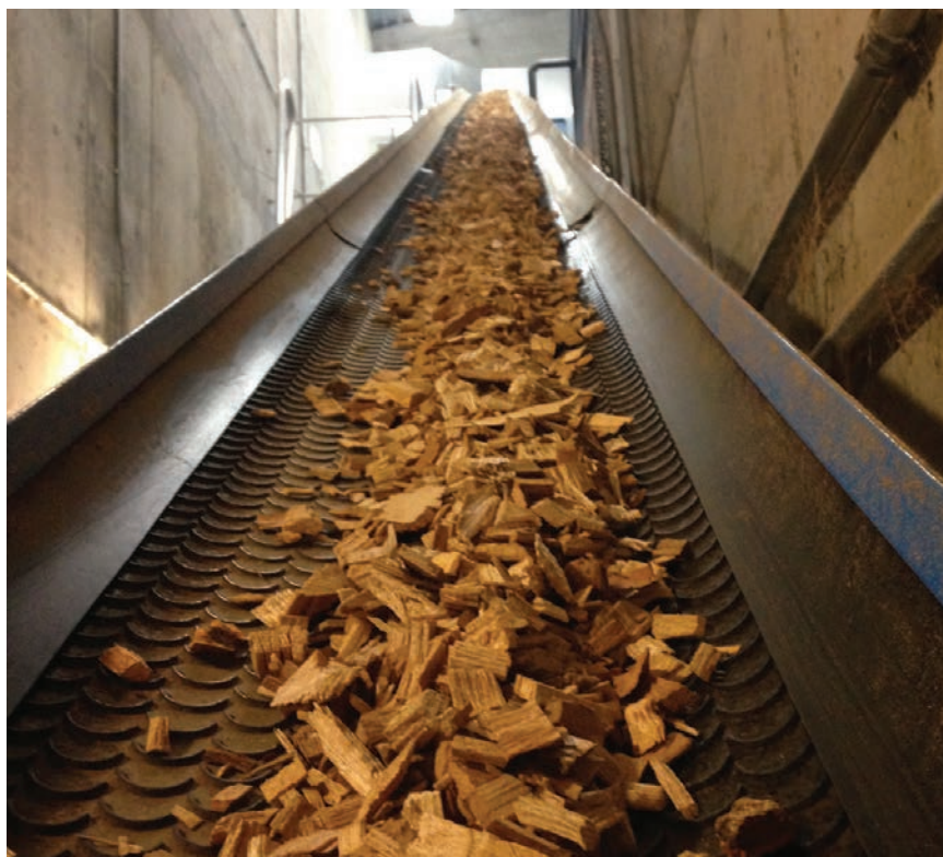
FIGURE 7: Woodchip fuel moving from storage to burner on a conveyor
