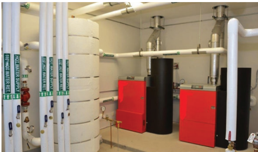
FIGURE 14: Example of two small pellet boilers (red) coupled with a thermal storage tank (large white insulated tank on left).
